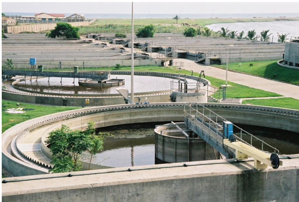
Figure 3: Sewage treatment plant, Accra
